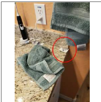
3rd Floor, RIGHT FRONT Bathroom (Missing grout)
