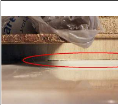
3rd Floor, RIGHT REAR Bathroom (Gap in caulking / grout)
