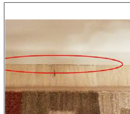
3rd Floor, RIGHT REAR Bathroom (Gap in caulking / grout)
