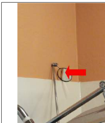
3rd Floor, RIGHT FRONT Bathroom (Gap in caulking coverage)
