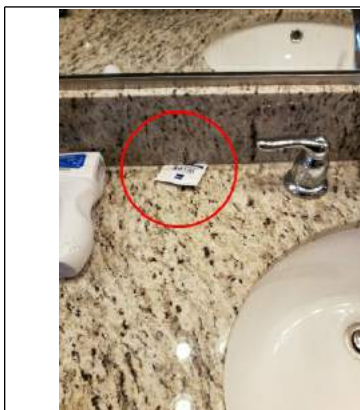
3rd Floor, RIGHT FRONT Bathroom (Missing grout)
