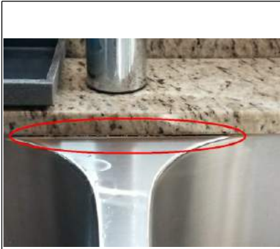
Gap in caulking coverage
