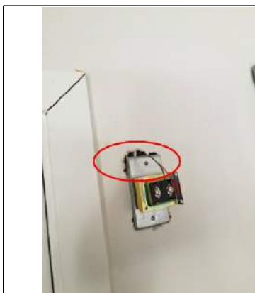
Hole in GARAGE wall
