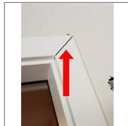
Separation in trim around GARAGE door
