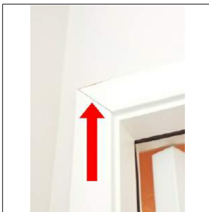
Separation in trim around GARAGE door
