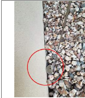
Weep screed hole
